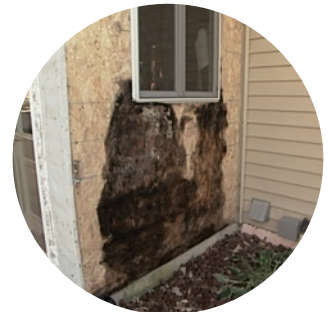
House rot from improper moisture management
