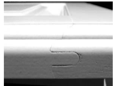
Example of end joint separation
