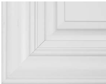
Example of front joint separation
